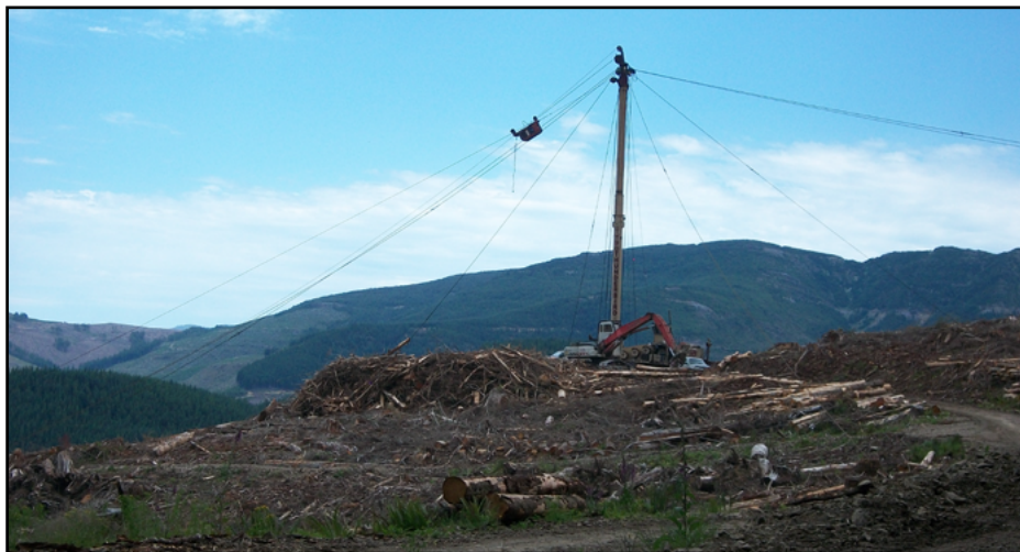
Figure TPO-3.4. Skyline yarder with radio-controlled carriage (Photo by Eric Simmons, BBER).
